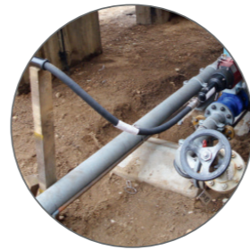
ANLAGENBAU PROCESSING INDUSTRY
